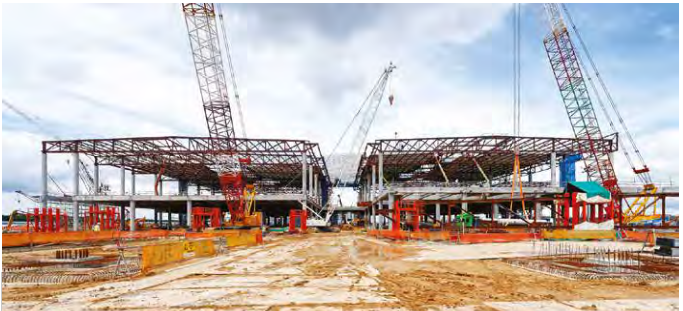
The sloping top-chord pitched trusses supporting the terminal roof were also prefabricated offsite.
