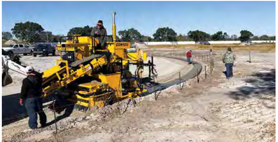
The new Gomaco Commander II two-track curb and gutter machine at work slipforming at the Banyan Cay Resort & Golf in West Palm Beach, Florida.
