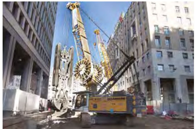
Liebherr HS 8100 HD with hydraulic slurry wall grab on Milan metro project.
