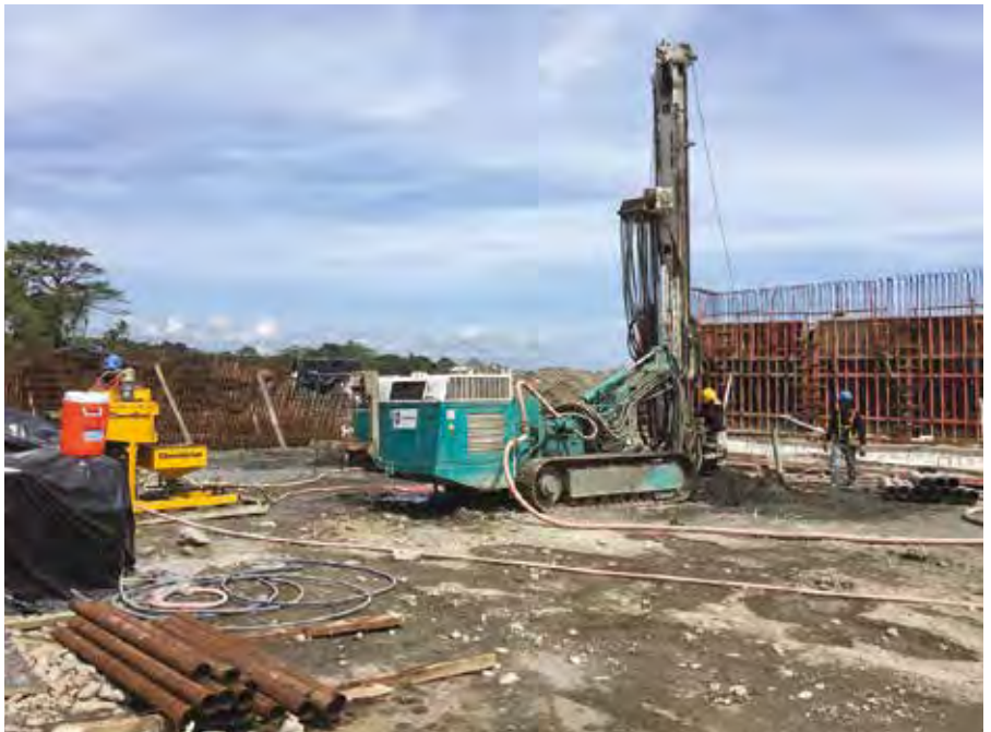
The CG-550/030 Rugged HP series is seen here (on the left) working on a foundation project. The machine can be skid-mounted or trailer-mounted, equipped with a 170-l mixing tank, 57-l or 113-l holding hopper and single-acting 3-in piston grout pump.
