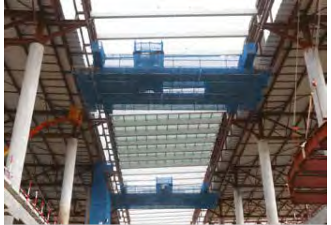
'Magic carpets' being used to install glass panels on the Galleria Skylight. These mobile hanging platforms were able to move along the entire roof safely.
