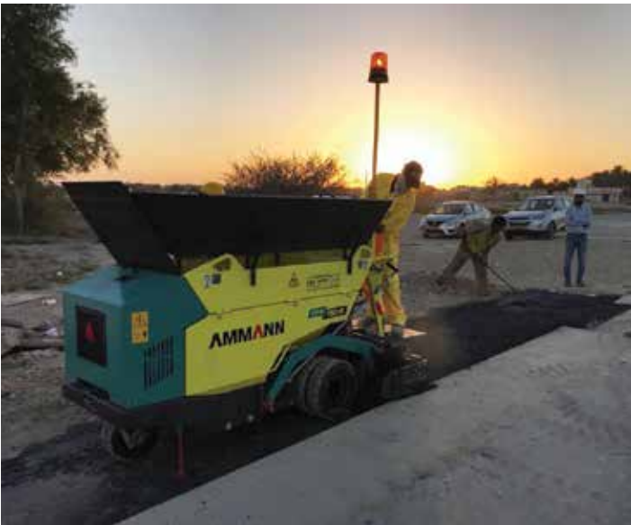
Ammann AFW 150-2 mini paver was recently used on a water pipeline installation project in Barka, Oman. Paving widths varied from 600 to 1,000 mm at different stretches and the flexibility of the paver provided significant advantages.
