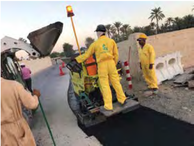
ABOVE: The paving work took about two months and involved placement of 4,000 t of mix. Spanning over 8 km, the project was designed to provide access to an improved water system for 130,000 residents.
