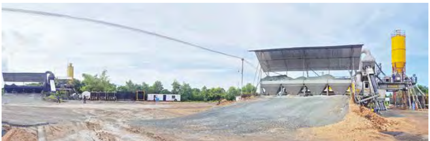
BELOW: Two Linnhoff TSD1500 mobile asphalt plants are currently in operation at the new Panglao Island International Airport to help build the runways and several roads on the project. Both plants are placed in close proximity to the jobsite, in order to maintain the strict requirement of the temperature for the hot mix asphalt.
