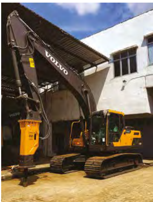
The Volvo EC210D excavator, fitted with a Volvo HB21 breaker, plays a key role in the construction of the access road to the new PLTA Batang Toru hydropower plant in Sumatra, Indonesia.
