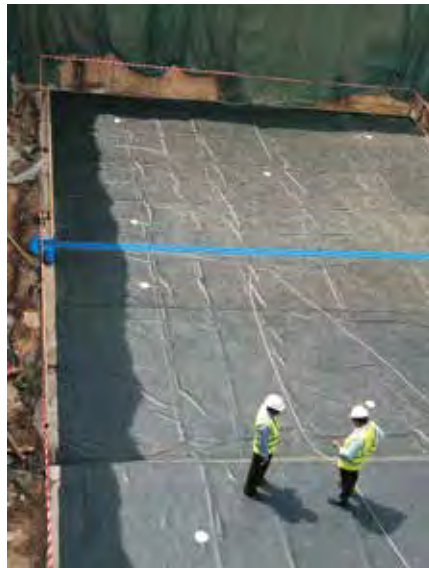
ABOVE: Mapei provided its waterproofing solutions for the Line 3 of Riyadh Metro, including Mapeplan TU S and Mapeplan PVC Protection 15 membranes, as well as Mapeplan injection valves, among others.
