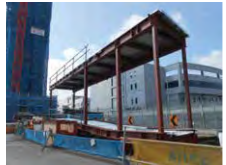
Fixed gangways were prefabricated offsite and assembled onsite – two at a time and without any welding works. This method improved productivity in general.
