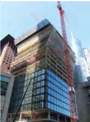
LEFT: The protection screen developed by Doka can be tilted 21° forward, backward and also to the side. BELOW: From level to level at the spiralling offset, the building steps up to 1.35 m round the perpendicular.
