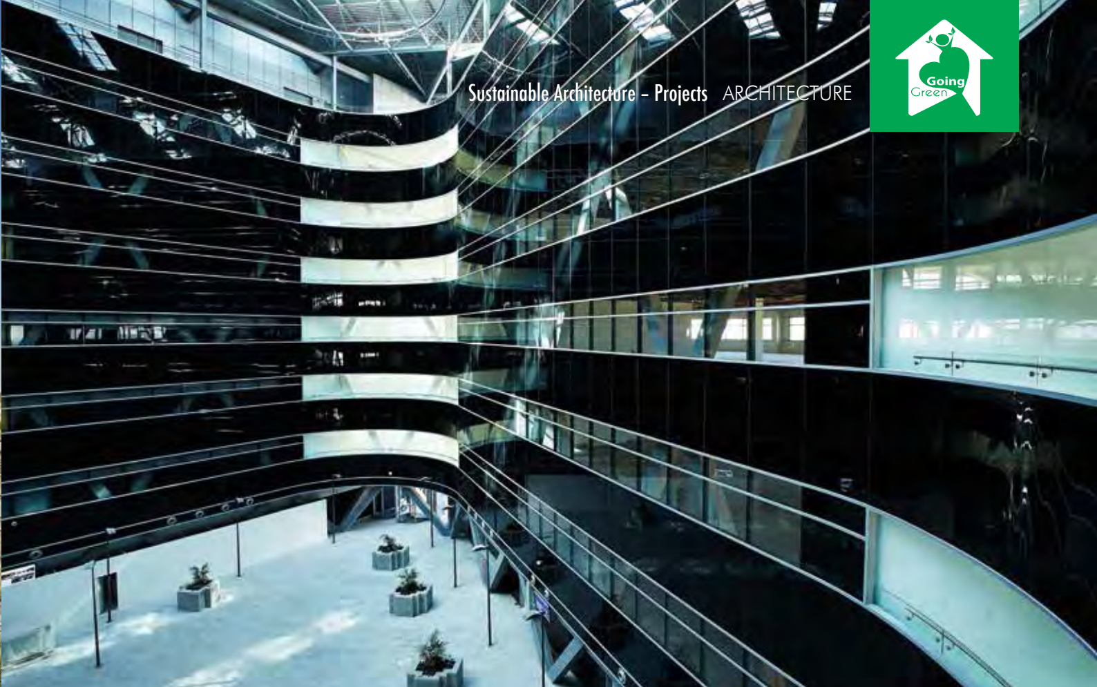
Interior of the IRENA headquarters. The air-conditioning system recovers 75 percent of the energy released through air exhaust, using this to cool incoming fresh air. Photo: © International Renewable Energy Agency (IRENA)
