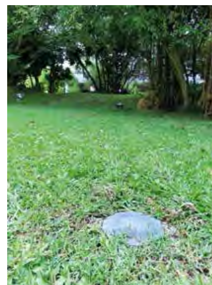
Fig 10: The vertical drain that attracts surface run-off is cleverly camouflaged within the turfed area and valleys of the roof garden.
