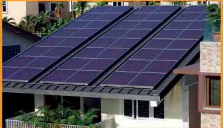
Residential Rooftop - 8.58kWp, Singapore
